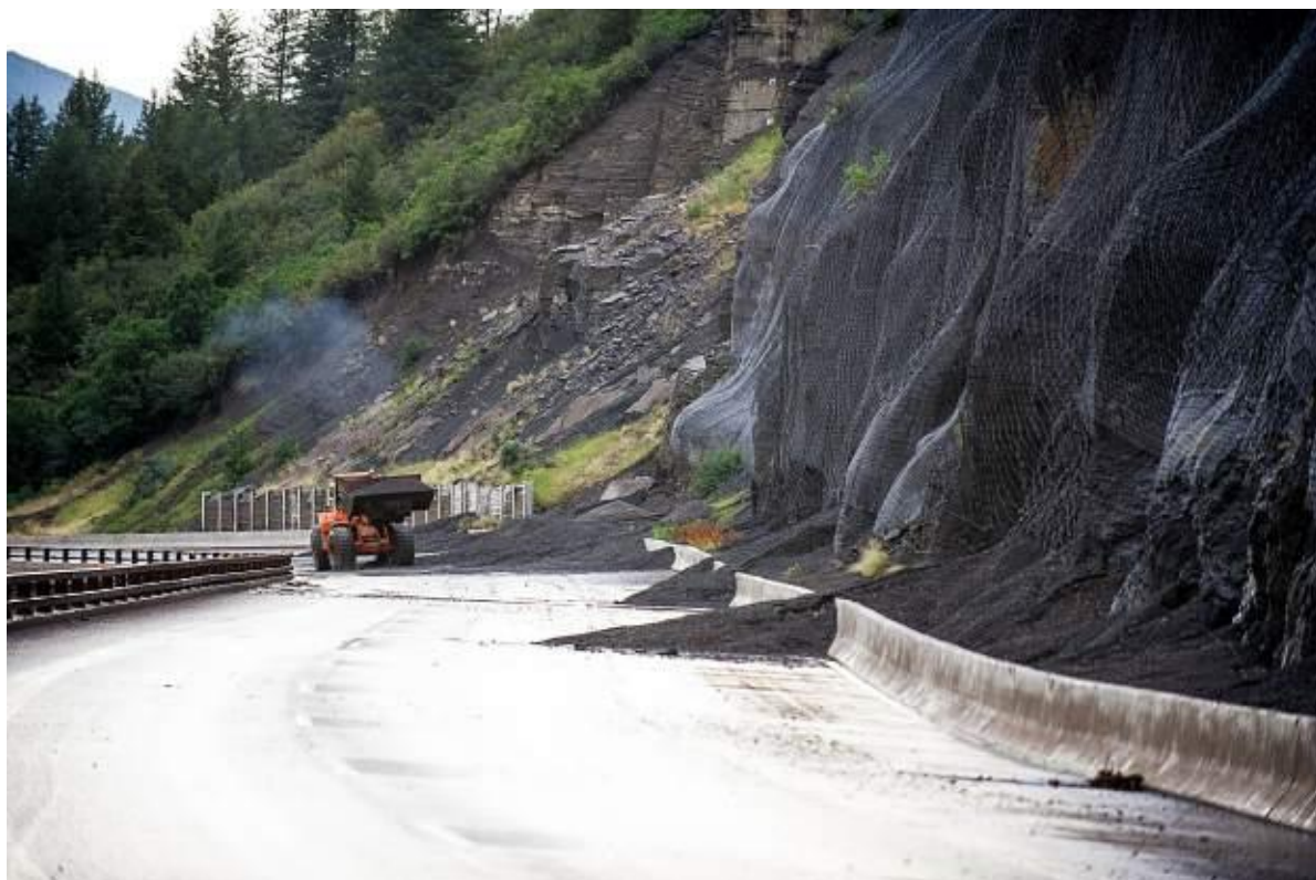
Figure 4-27 Rockslide on Highway 82 Near Aspen on July 11, 2017
